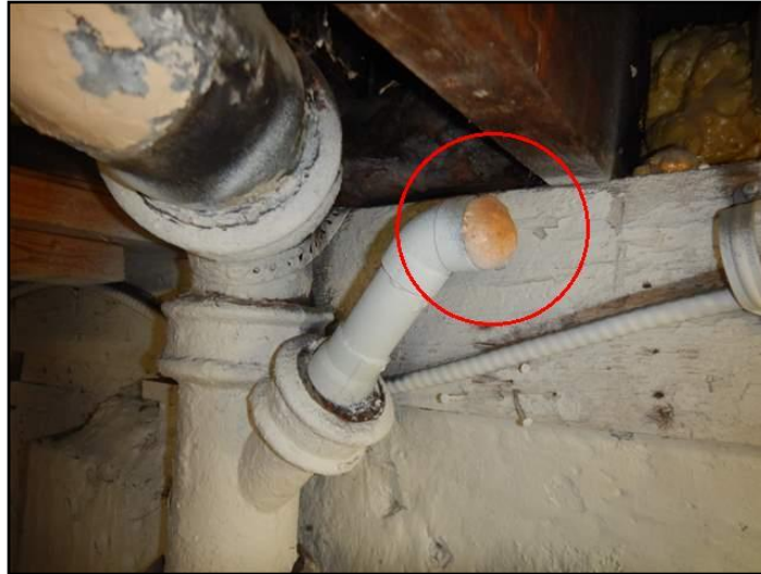
Unsealed pipe openings
