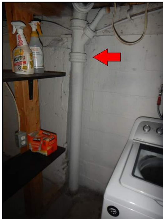
Cast iron waste stack
