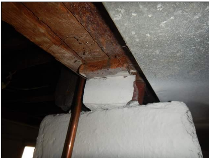
Poor bearing, crushed or loose shims
