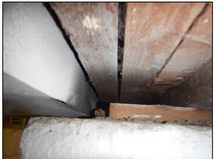
Poor bearing, crushed or loose shims
