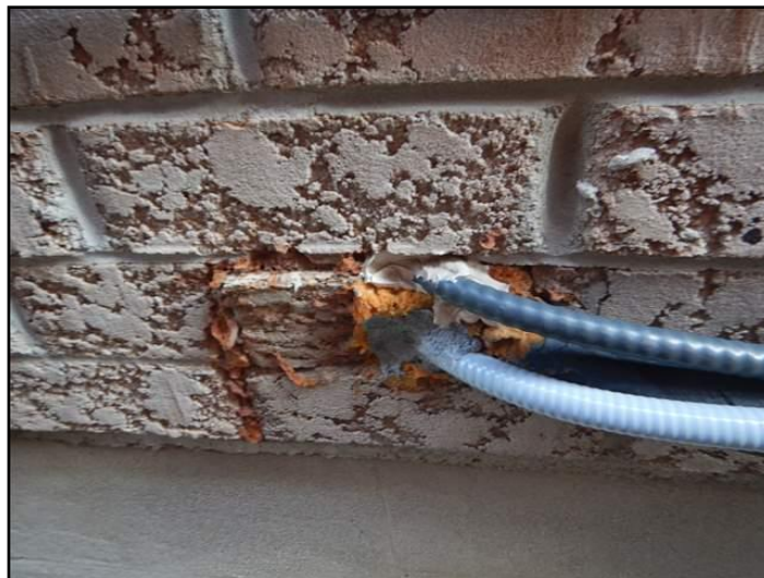
Poor seal at building
