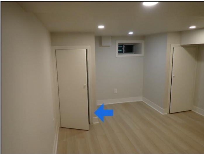
Main water shutoff
