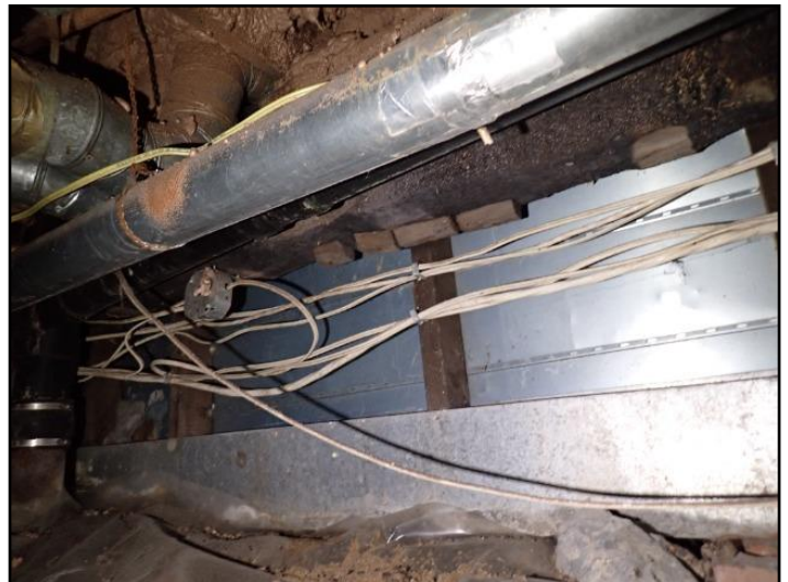
Ex. Fire damaged beam
