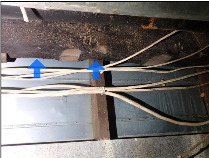
Ex. Fire damage - charring
