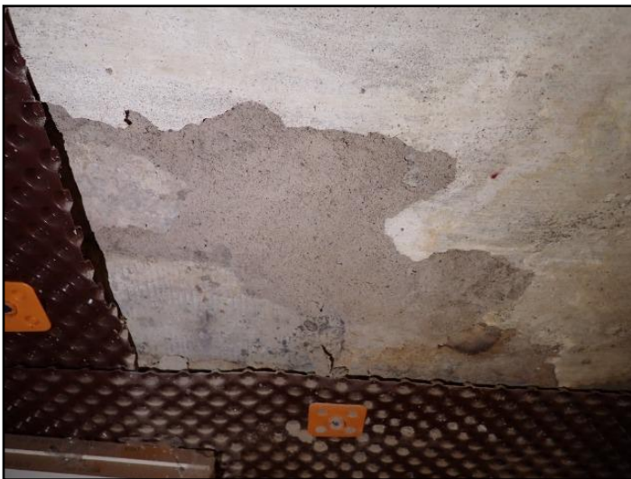
Ex. Sump pump area
