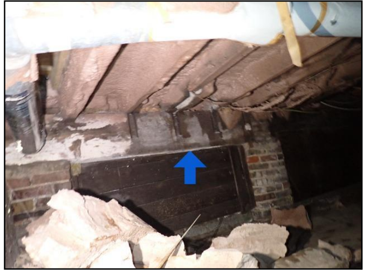
Ex. Moisture damage / rot
