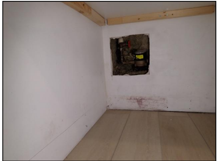
Main water shutoff
