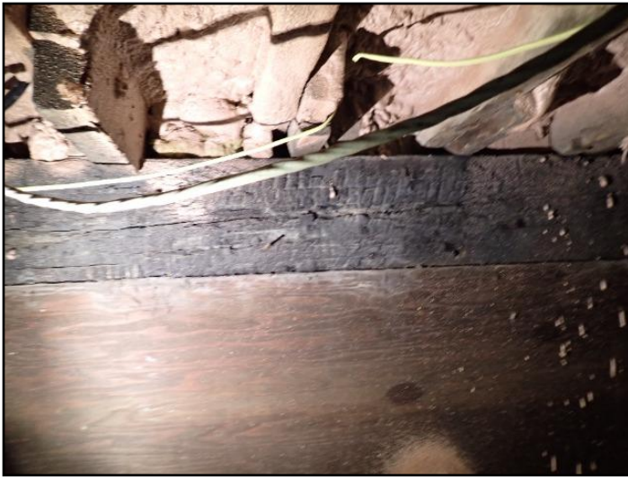
Ex. Fire damaged beam
