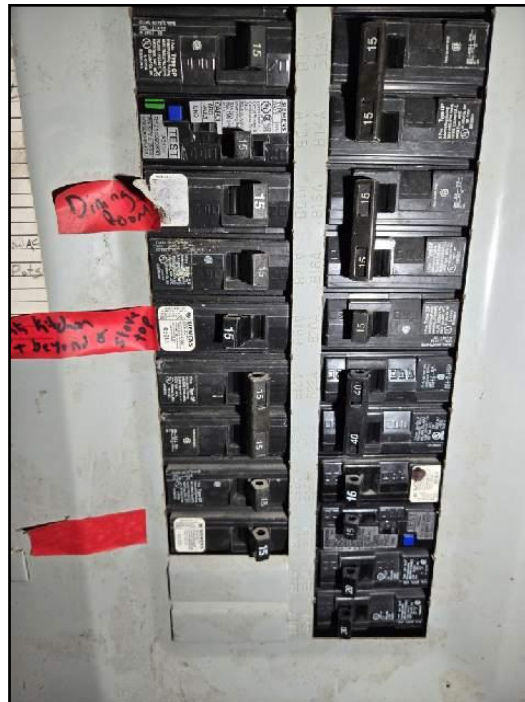
Breaker in OFF position
