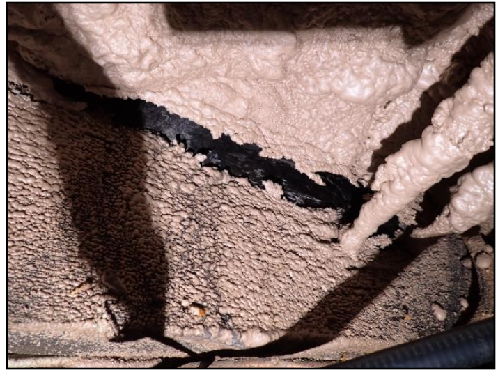
Crack in spray foam - Fire damage underneath
