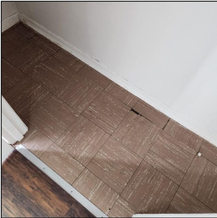
38. Possible asbestos containing materials
