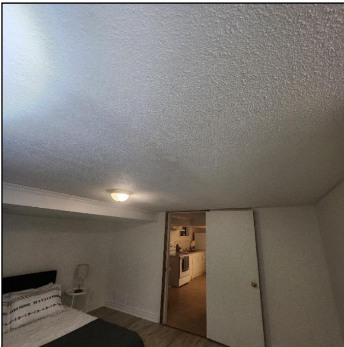
36. Possible asbestos containing materials
