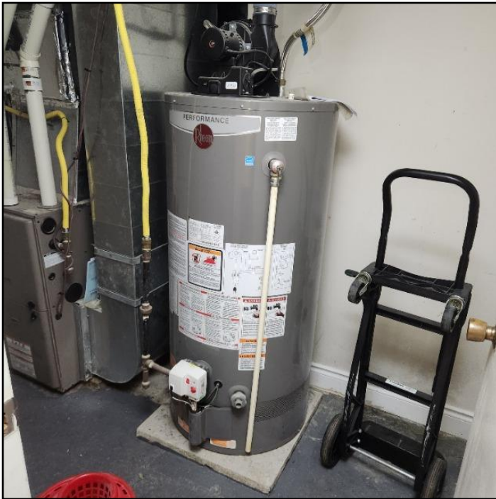
19. Conventional hot water tank
