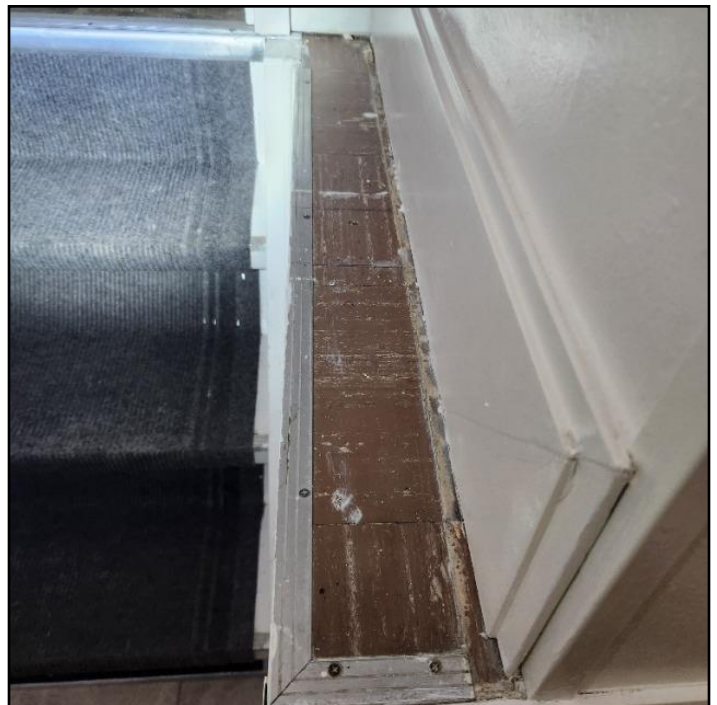
37. Possible asbestos containing materials
