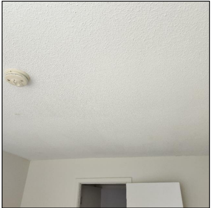
39. Possible asbestos containing materials
