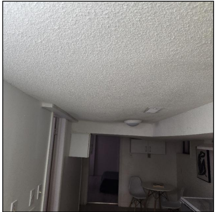
35. Possible asbestos containing materials
