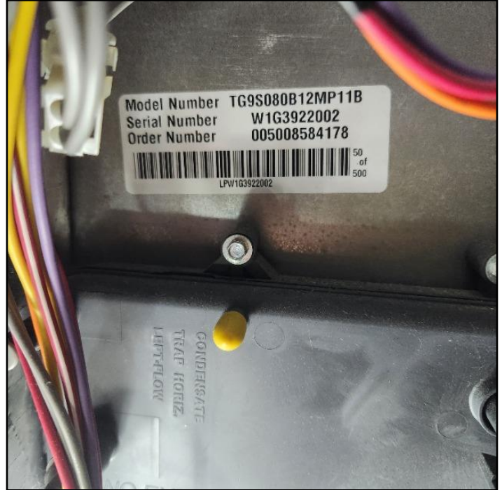
11. Furnace data plate
