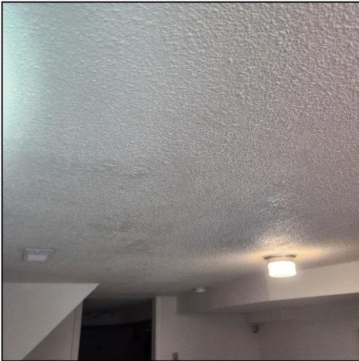
34. Possible asbestos containing materials
