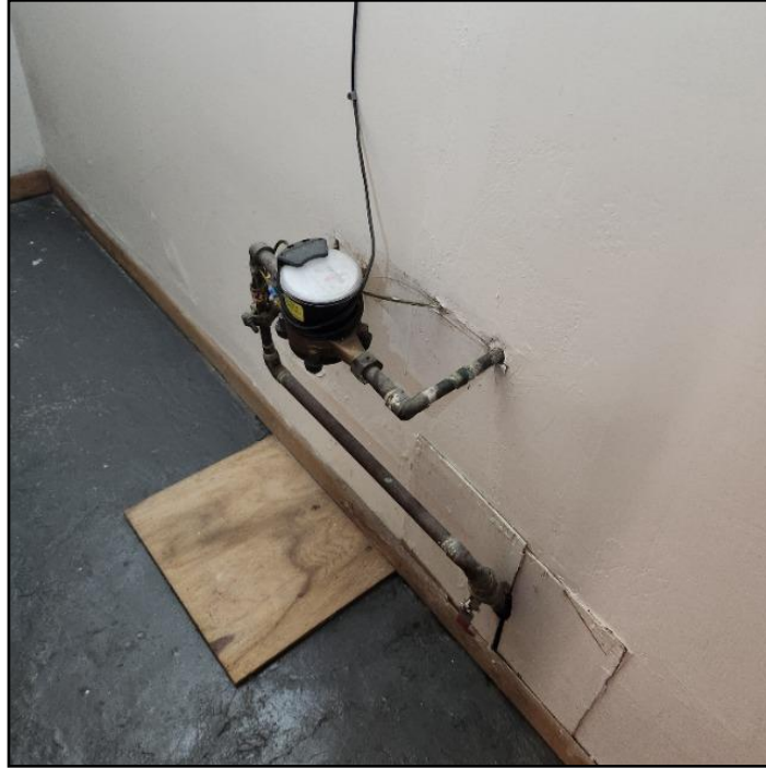
18. Main water shutoff
