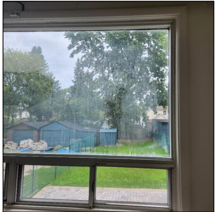
29. Lost seal (Interior View)
