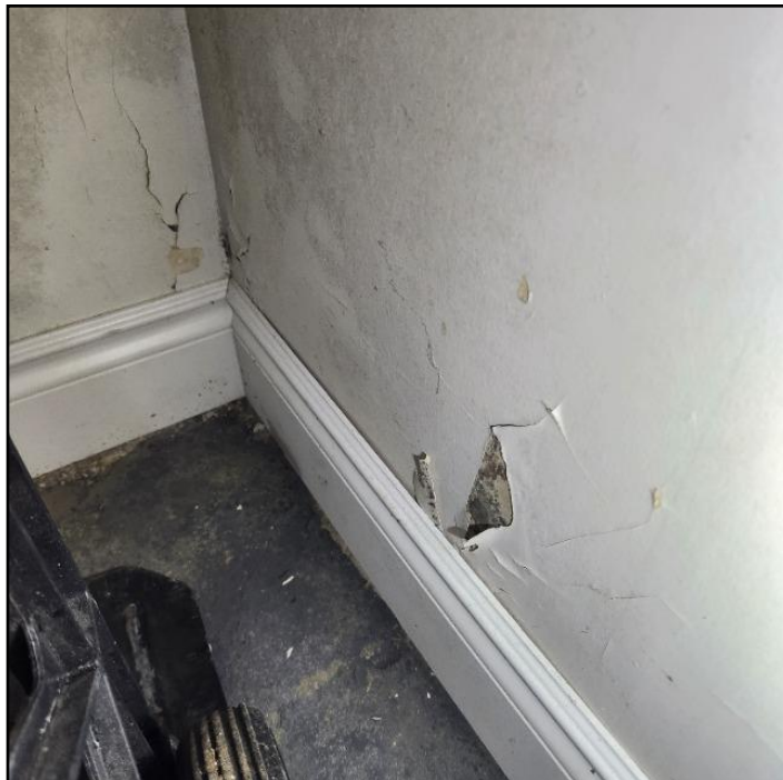
42. Mold at furnace room wall
