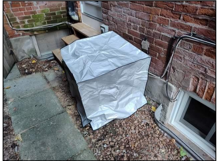
Air cooled condenser
