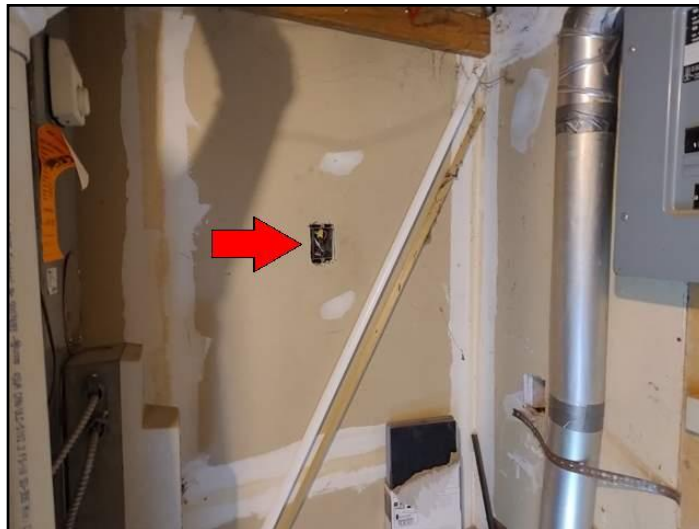
Missing cover plate
