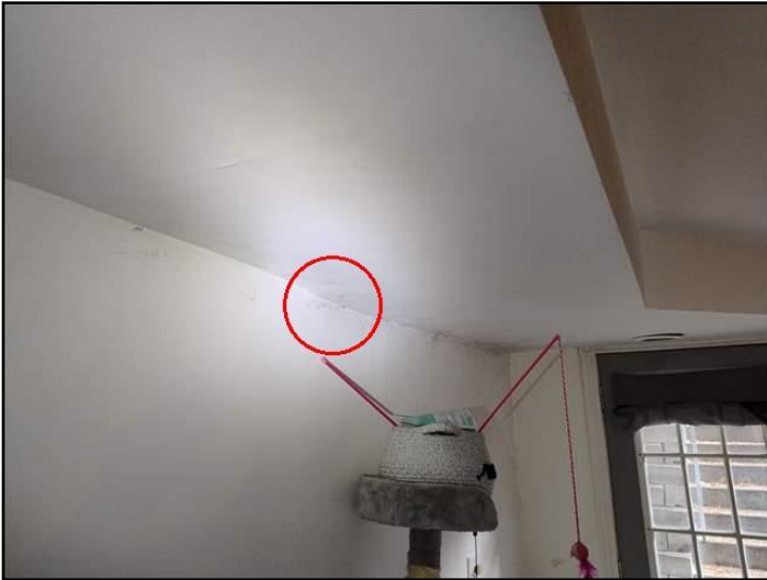
Water damage / patch
