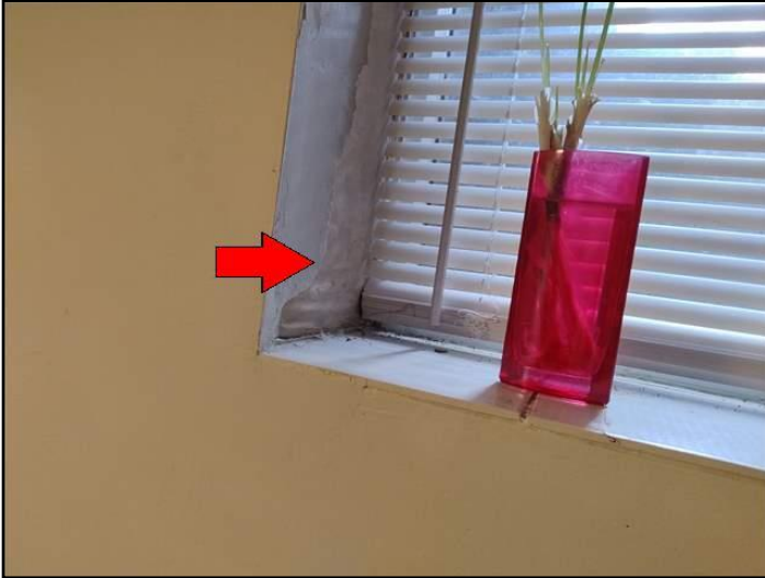
Ex: Water damage
