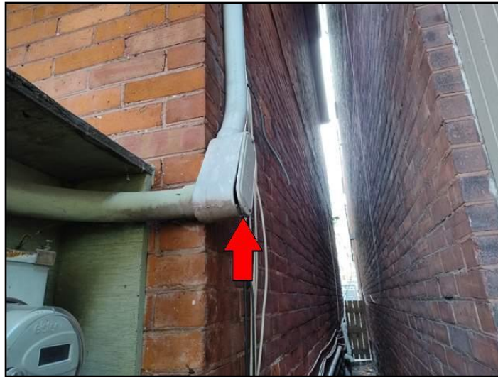
Cover not well sealed
