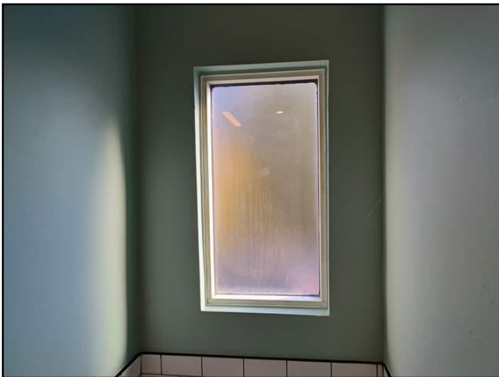
Ex: Evidence of condensation due to lost seal
