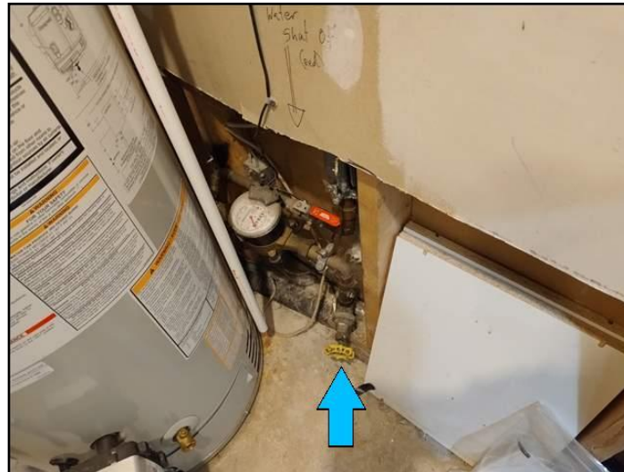
Main water shutoff valve
