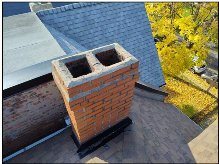
Rain caps missing
