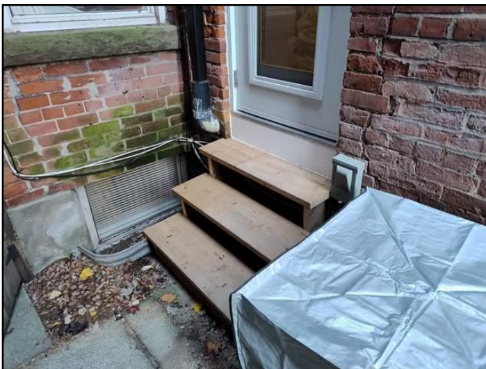
Ex: Missing handrail
