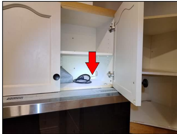
Extension cord used as permanent wiring
