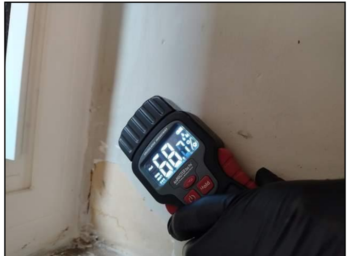
Close-up: High moisture
