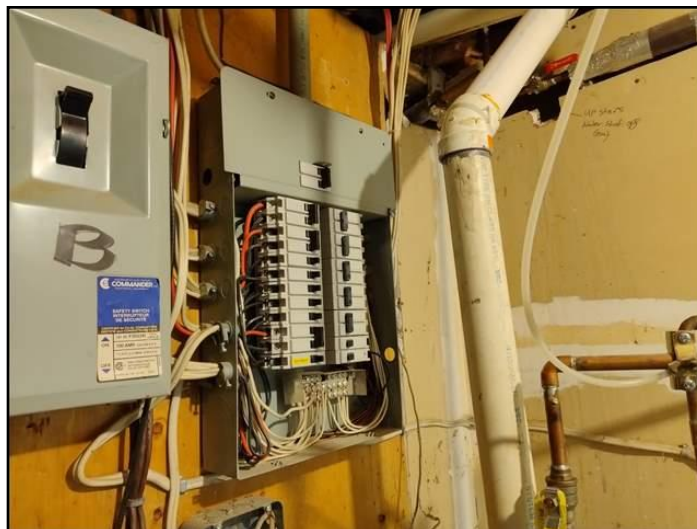
Breaker panel (cover removed for inspection)
