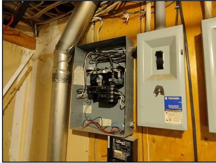
Breaker panel (cover removed for inspection)
