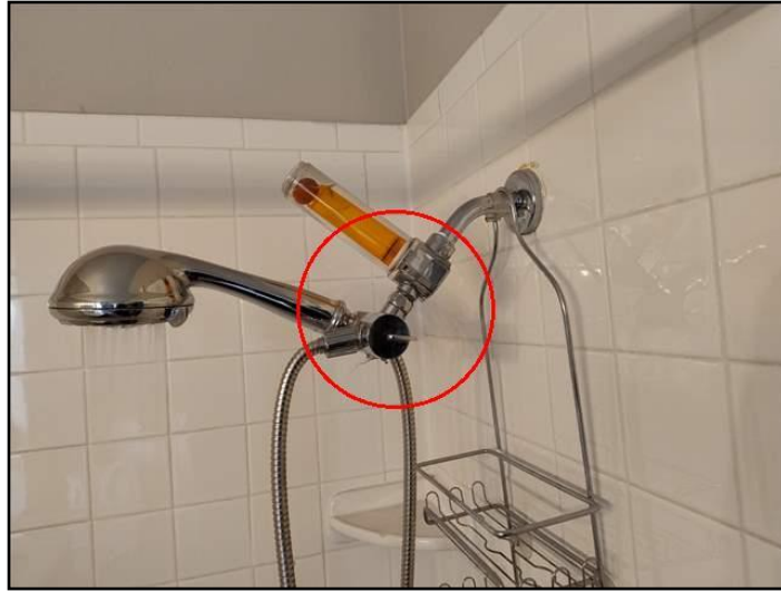
Leaky hand shower connections
