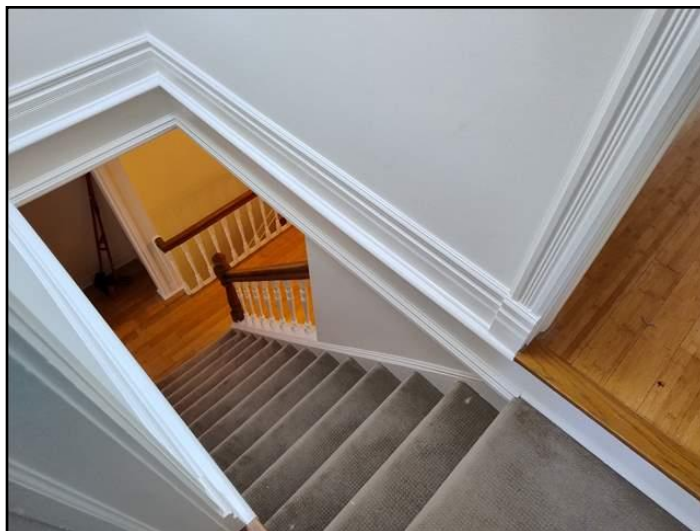
Ex: Incomplete or not continuous railing
