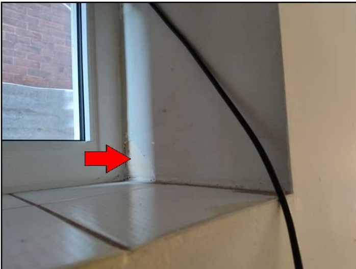
Ex: Water damage
