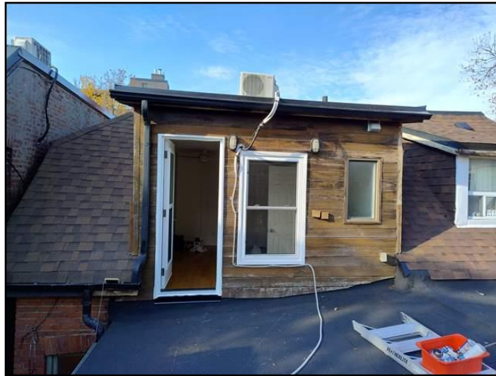
Unrestricted access to rooftop
