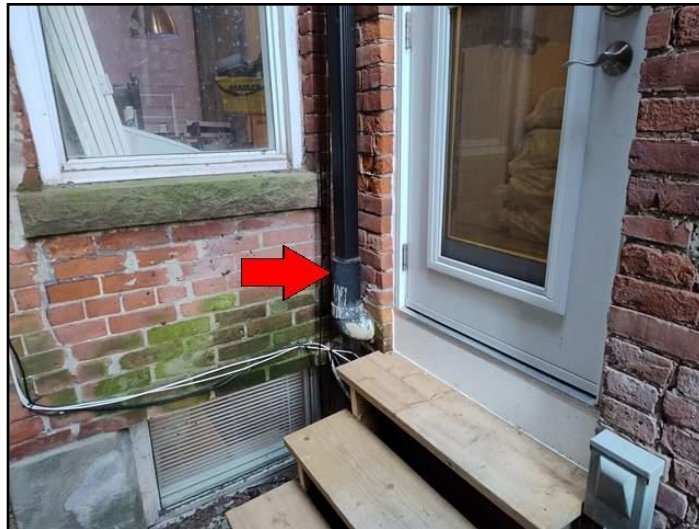
Discharges below grade
