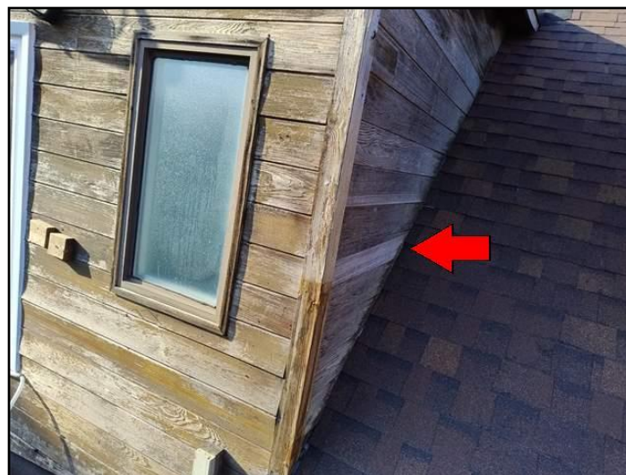
Ex: Siding too close to roof
