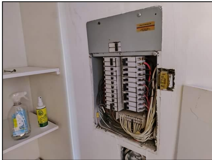
Breaker panel (cover removed for inspection)
