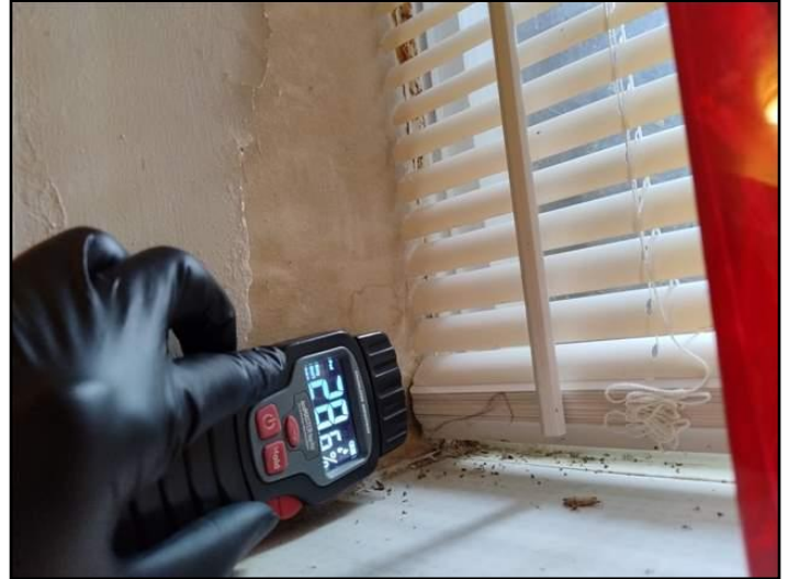
Close-up: Mid-range moisture reading
