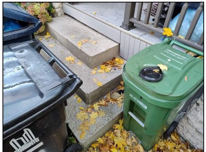
Ex: Missing handrail
