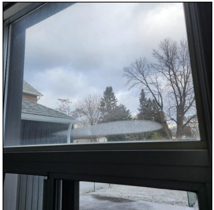
34. Lost seal on double glazing
