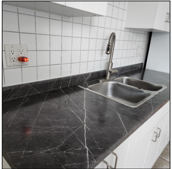
13. upgrade plug to GFCI
