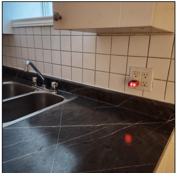
15. upgrade plug to GFCI
