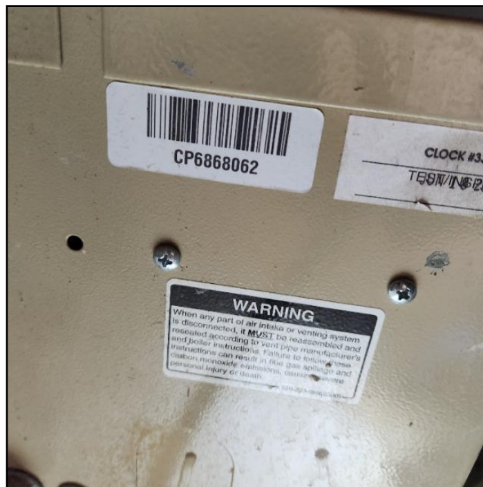
20. Boiler Serial Number
