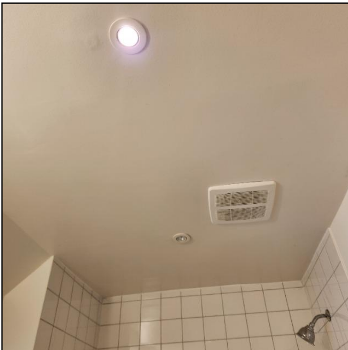
14. Light requires replacement
