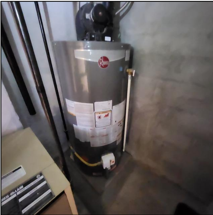
25. Conventional Hot water Tank
