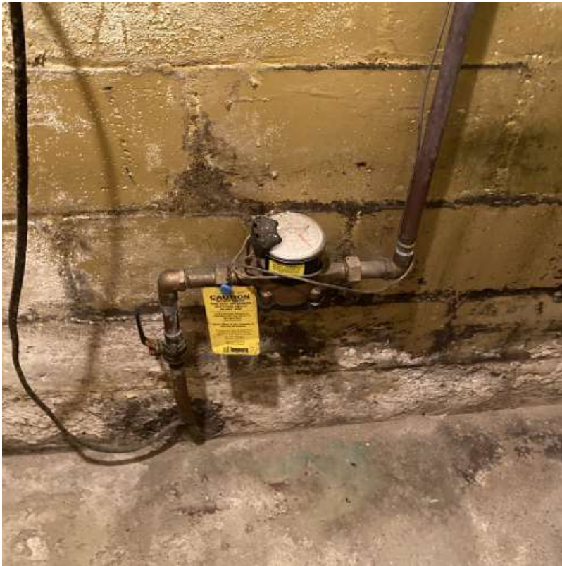
A view of the main water shutoff valve requiring possible heating repair.
