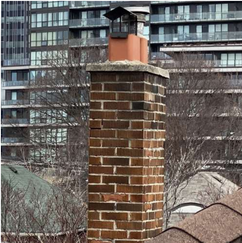
A view of the masonry chimney requiring repair.
