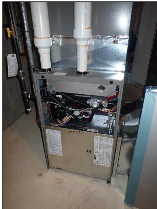
Furnace cabinet is in good condition
