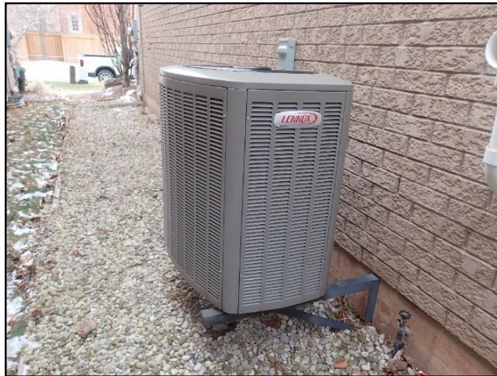
Air conditioner is approximately 5 years old
