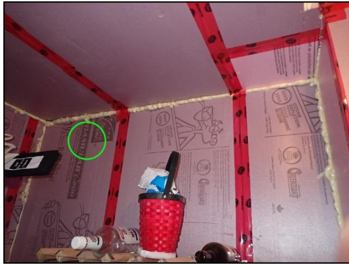
Cold Room vent(s) missing/not visible
