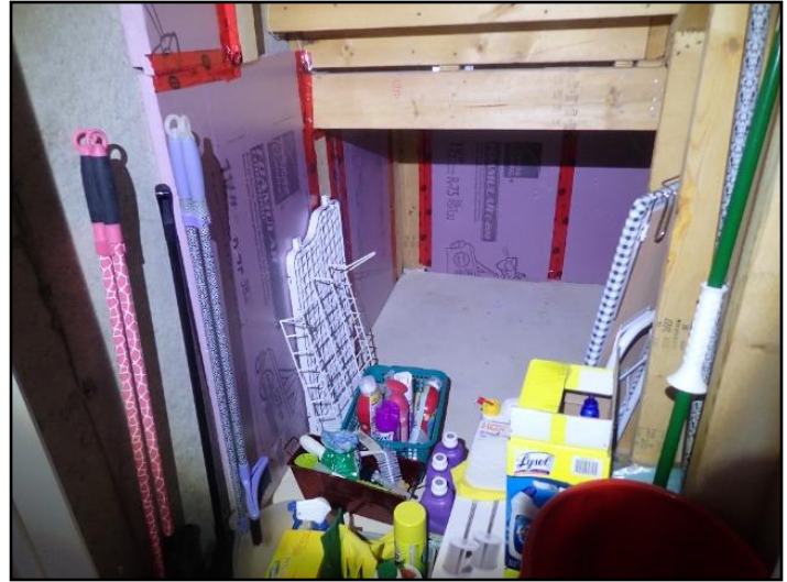
Exposed combustible insulation under stairs
