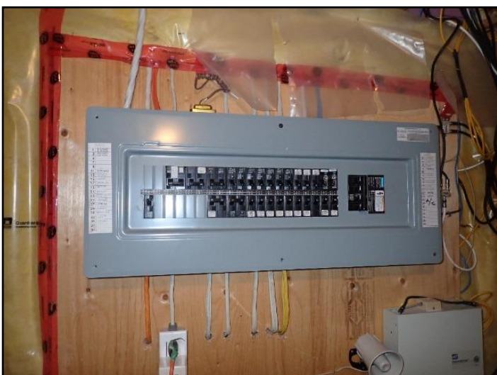
Panel and wiring are in good condition
