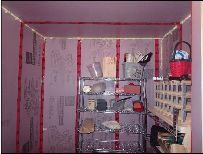
Exposed combustible insulation in Cold Room
