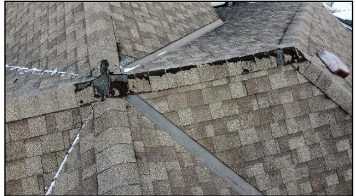
23. Missing, loose or torn
