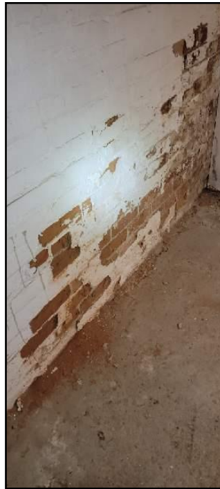
45. Spalling concrete or brick
