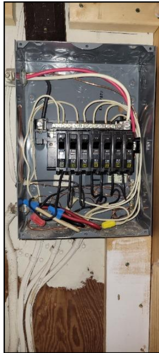
48. Breakers - first floor
