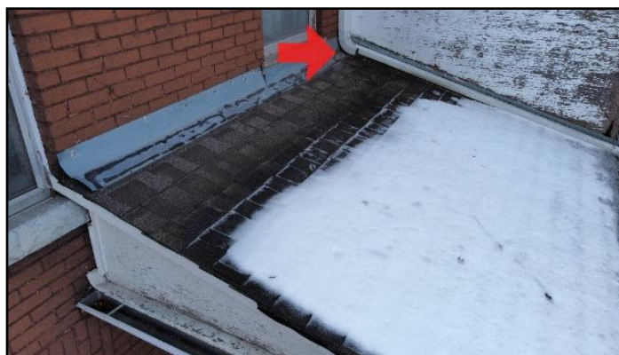
31. Discharge onto roofs
