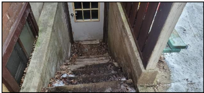
39. Guard and handrail problems
