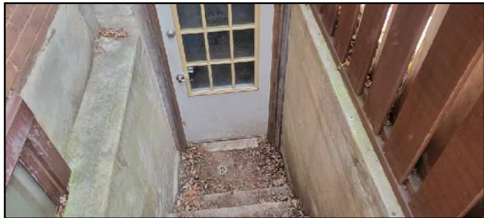
40. Door threshold missing, too low, not...
