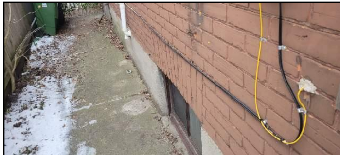
33. Too close to grade
