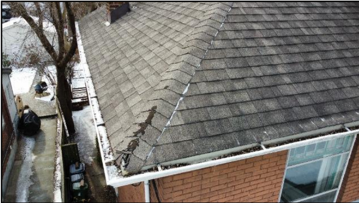
22. Missing, loose or torn
