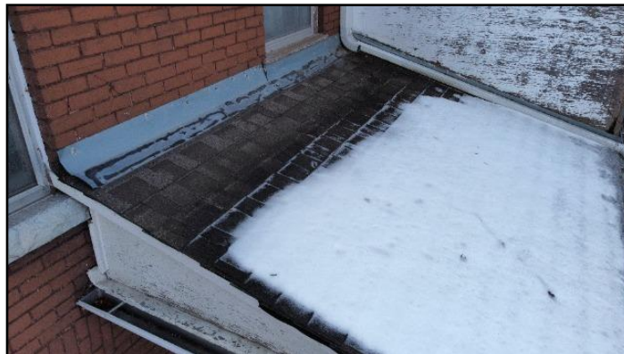
24. Damage, loose, open seams, patched
