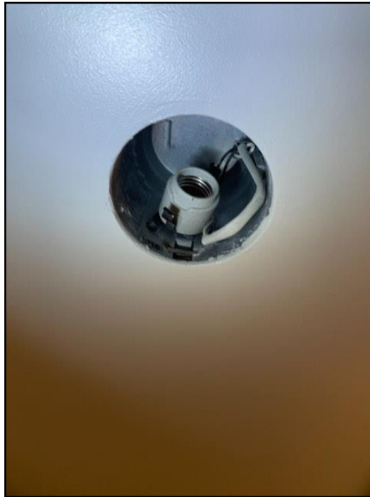
Missing light bulb and lens
