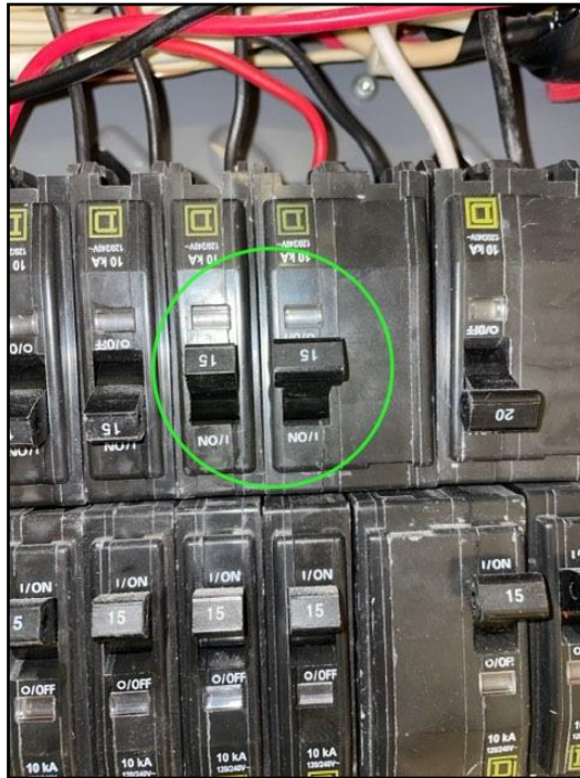
Breaker in OFF position
