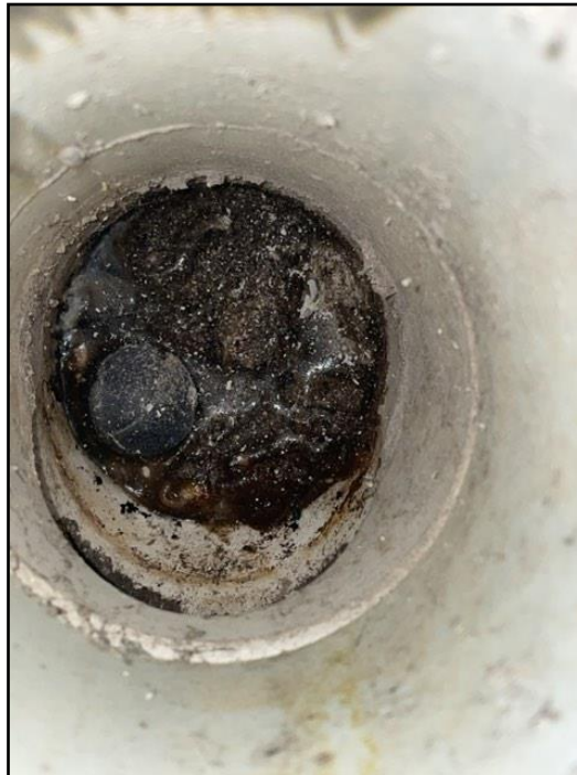
Debris in floor drain
