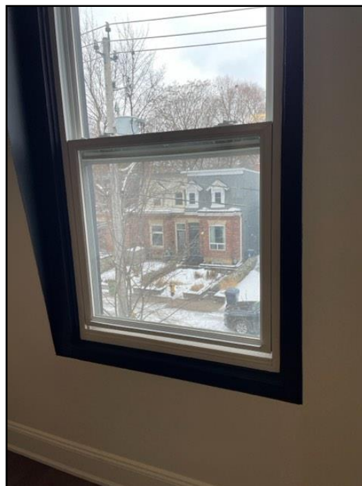
Difficult to operate
