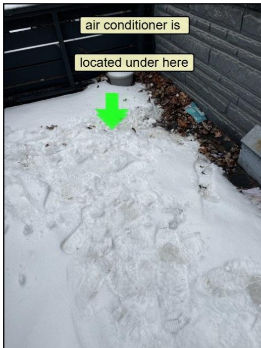
Data plate not accessible
