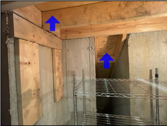
Wood forms not removed from concrete
