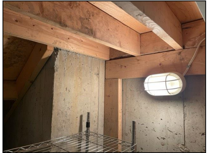
Wood forms not removed from concrete
