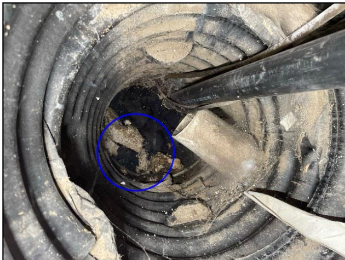
Debris in the sump, clogged sump
