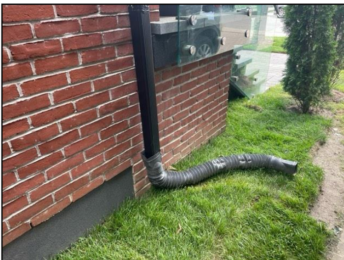
Discharge too close to building
