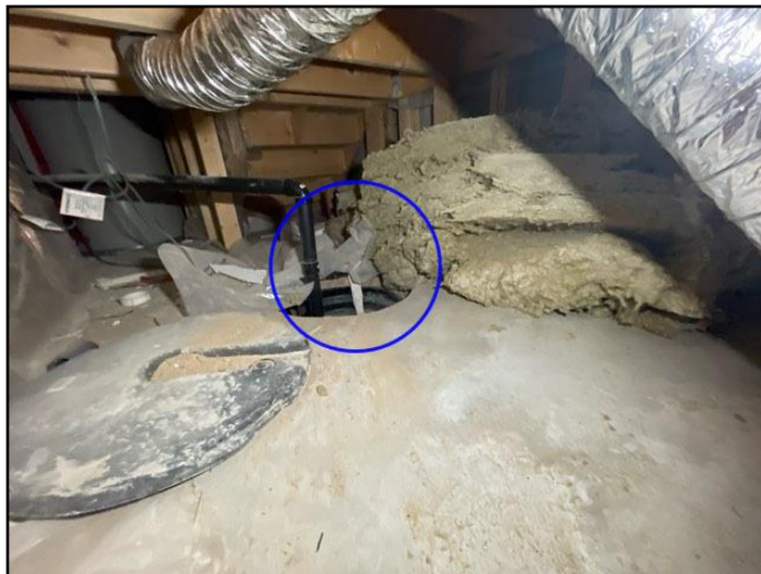
stored insulation - source of the debris
