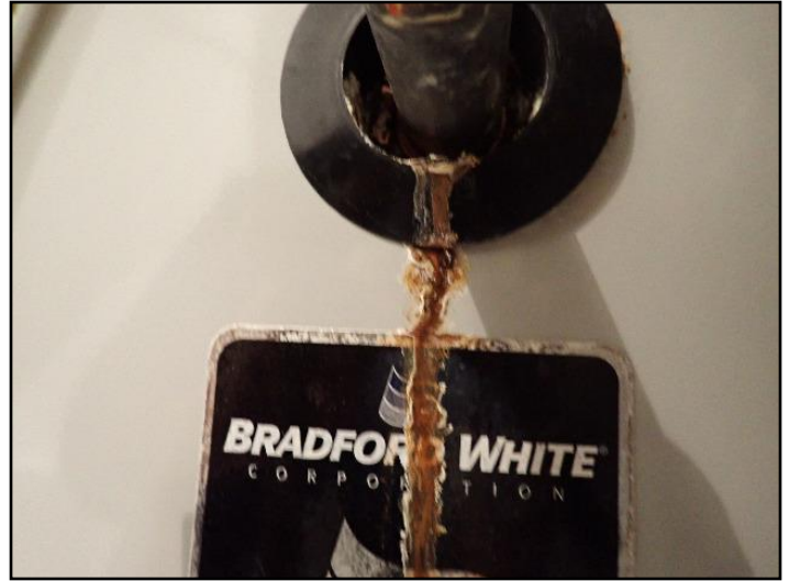
water stains and corrosion
