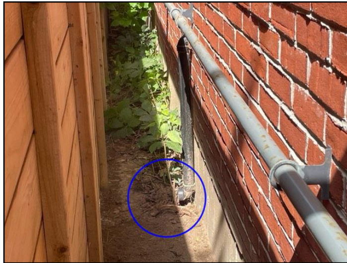
Discharges less than 6 feet from home
