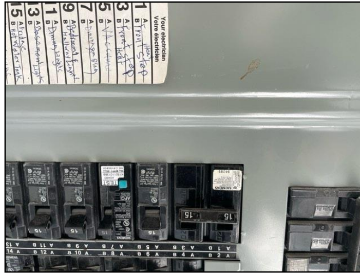
Breaker in OFF position
