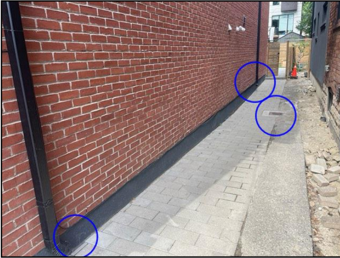
Discharge too close to building
