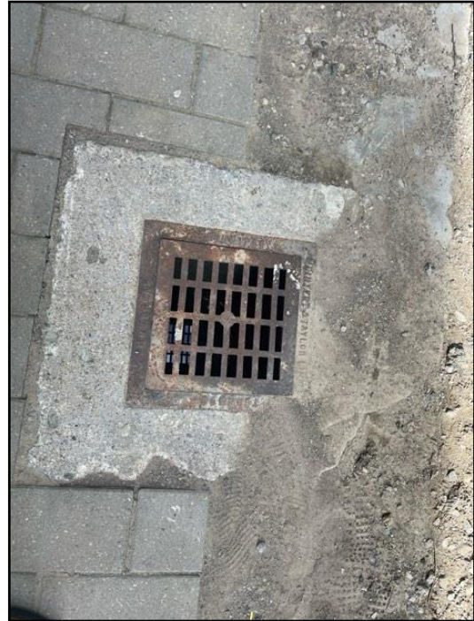
Drain / Catch basin
