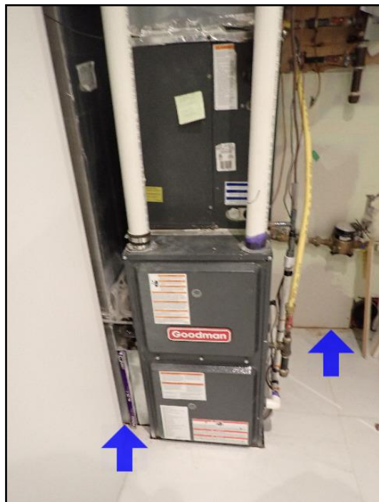
on floor under furnace
