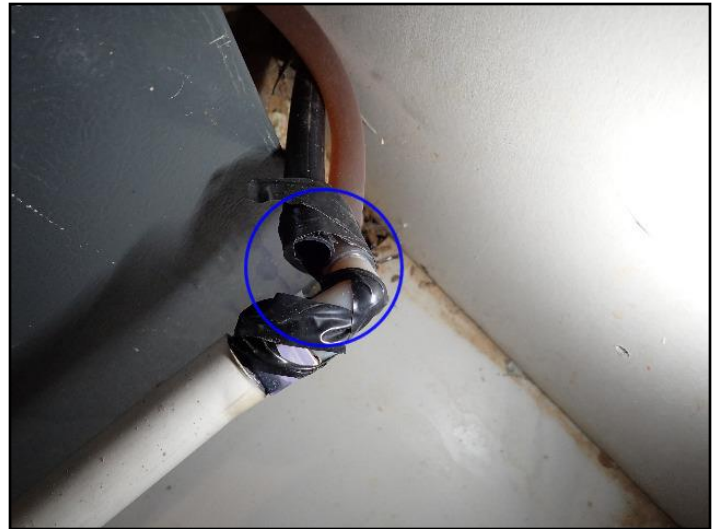
Condensate drain pipe
