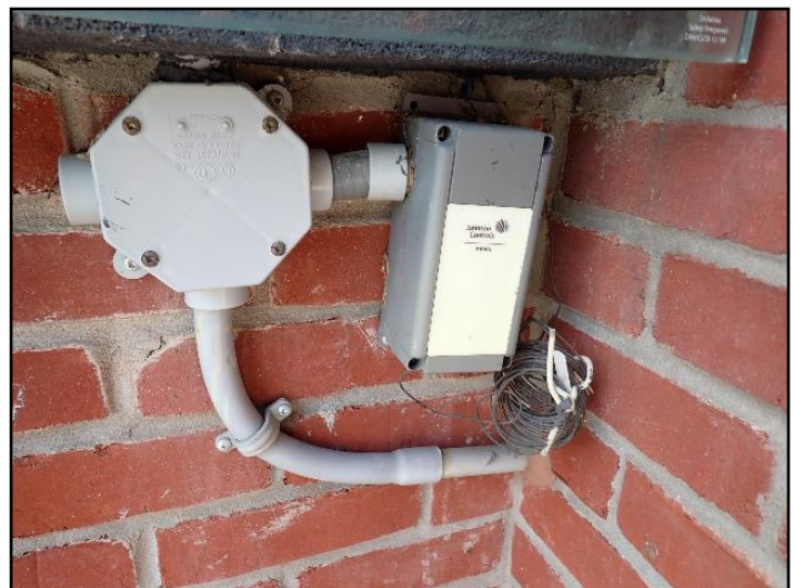
Junction and control box
