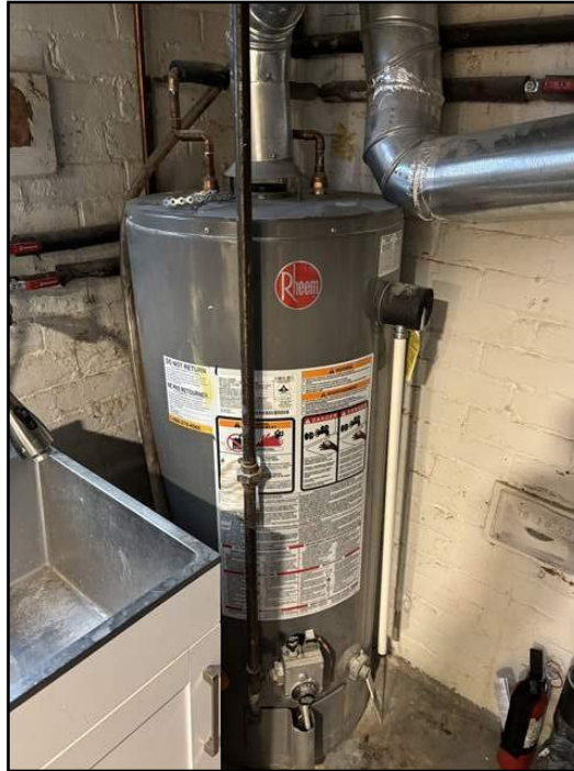
Water Heater near end
