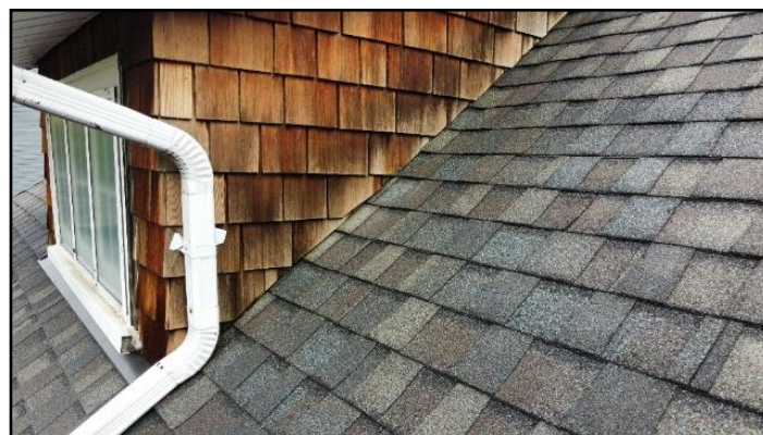
22. Siding not cut back
