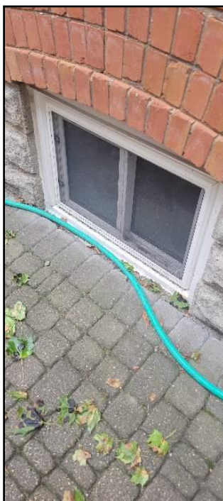
25. Too close to grade
