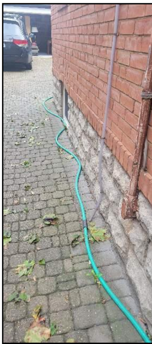
27. Unsealed gap at building
