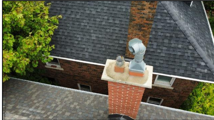
53. Rain cap missing or damaged
