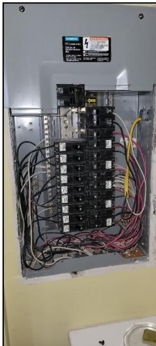
45. Breakers second floor
