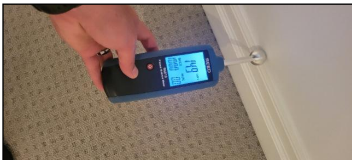
84. Moisture meter results
