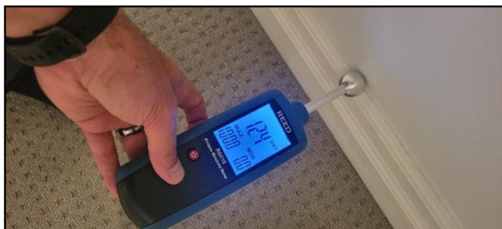
83. Moisture meter results
