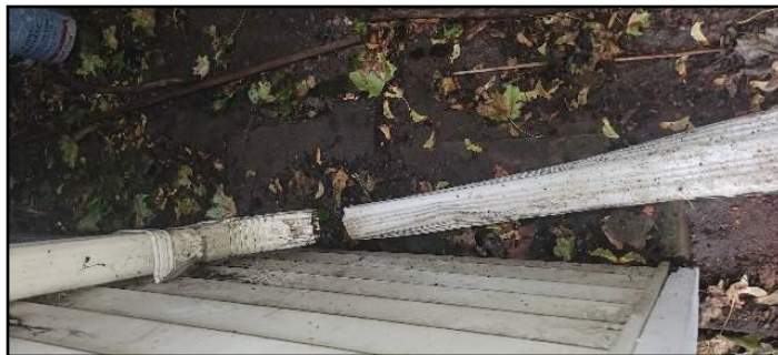
24. Discharge too close to building
