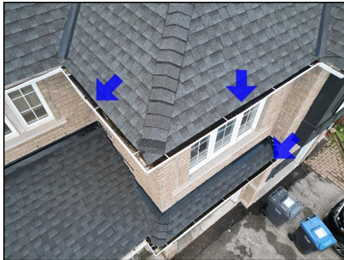
Improper slope, ponding
