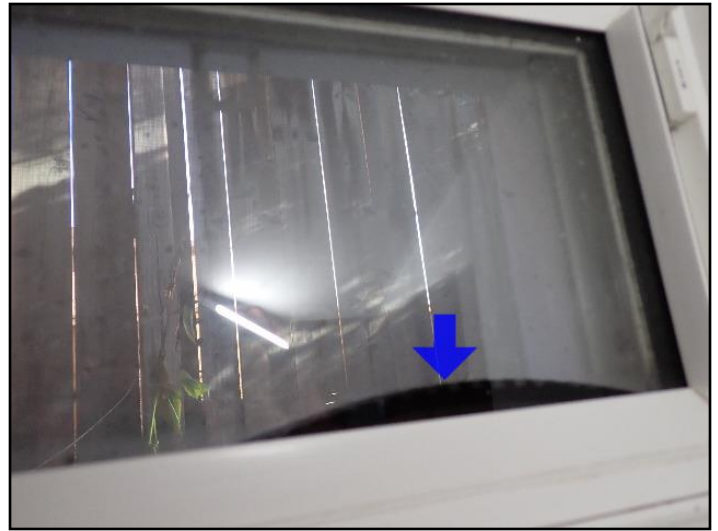
Basement window, swollen gaskets
