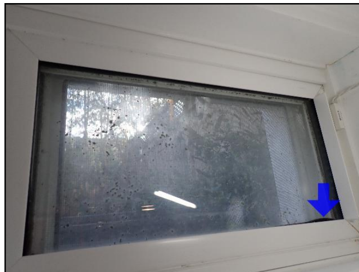
Basement window, swollen gaskets
