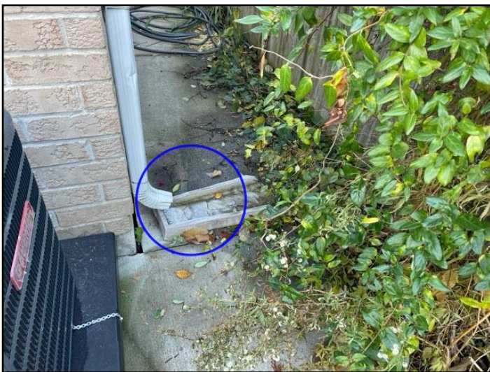
Discharge too close to building
