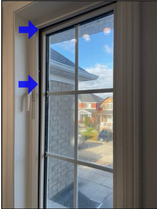
Window lock does not engage
