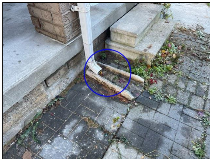
Discharge too close to building
