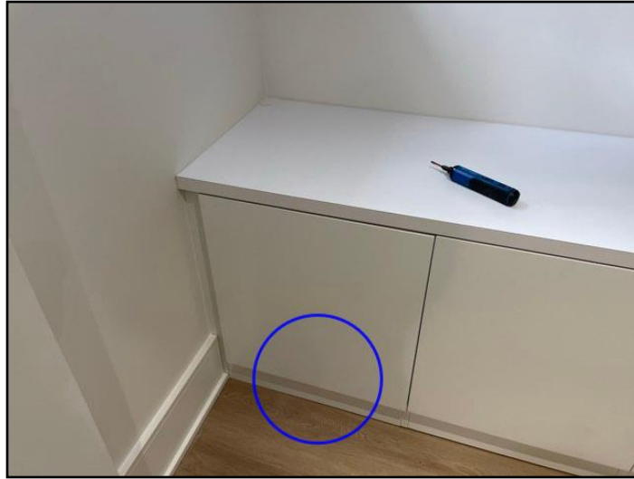
In basement cabinet
