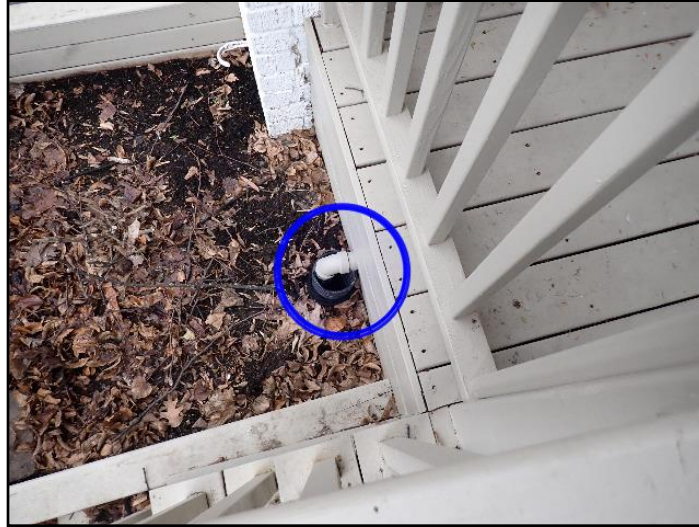
Discharges less than 6 feet from home
