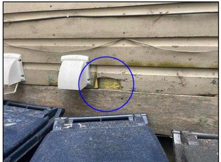
Cracked, split or broken
