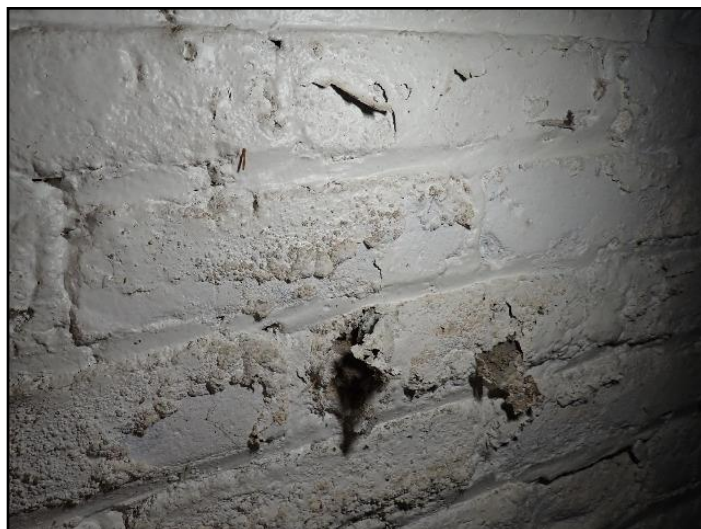
Efflorescence / Peeling paint
