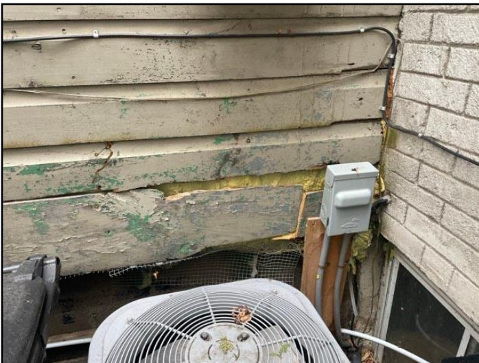
Cracked, split or broken
