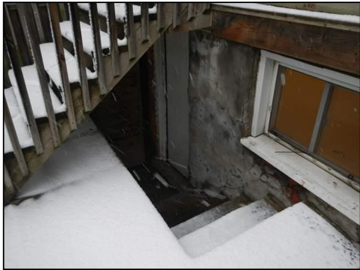
Guard / handrail - missing
