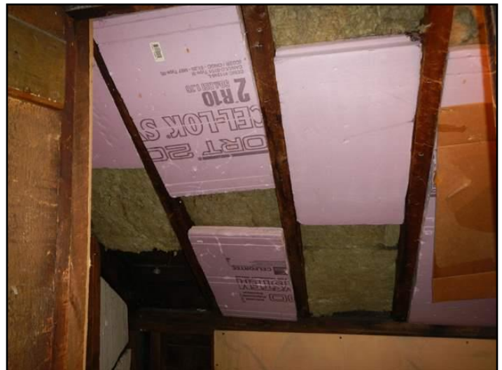
Exposed combustible insulation
