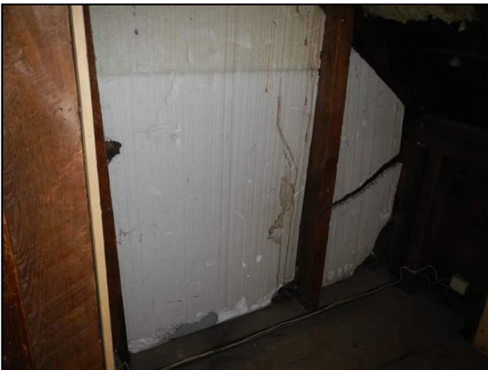
Exposed combustible insulation
