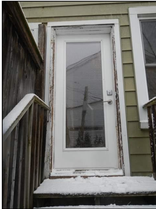
Paint or stain - needed
