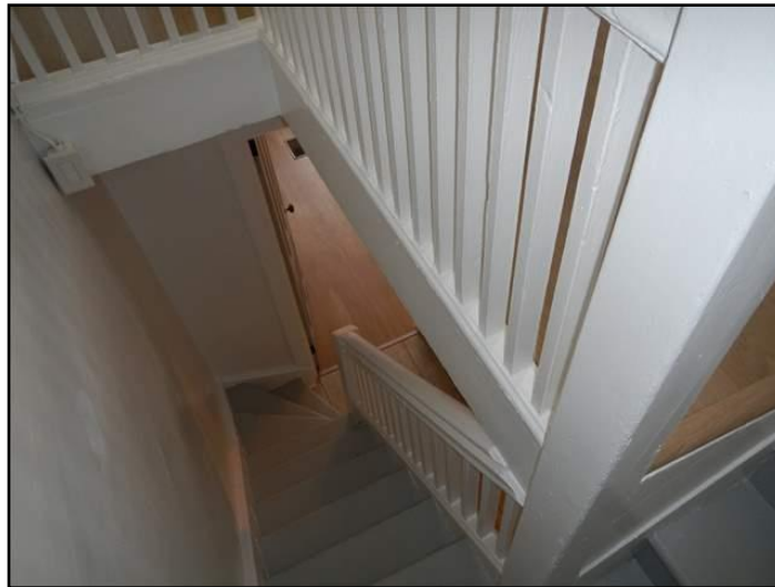
Incomplete or not continuous railing
