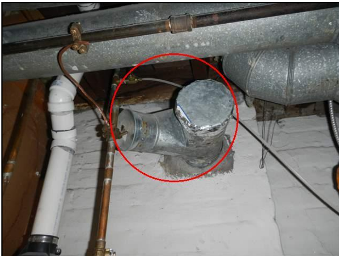
Blocked off in the basement
