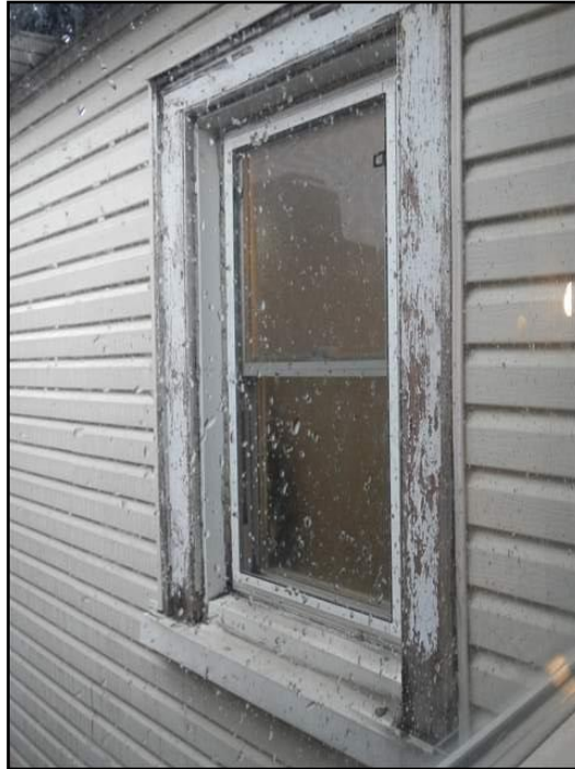
Paint and caulking - deteriorated / missing
