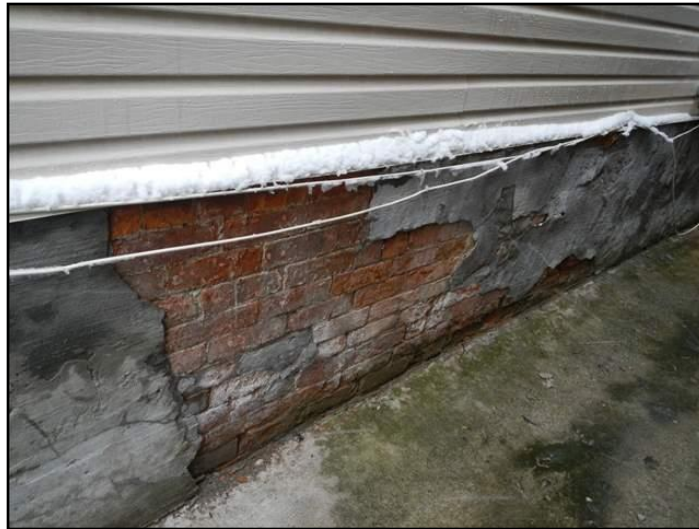
Parging damaged or missing
